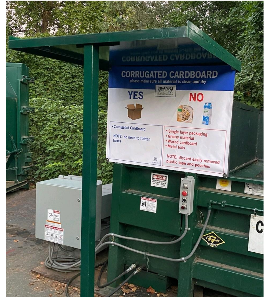
Corrugated Cardboard Compactor Control Station – McIntire Recycling Center
